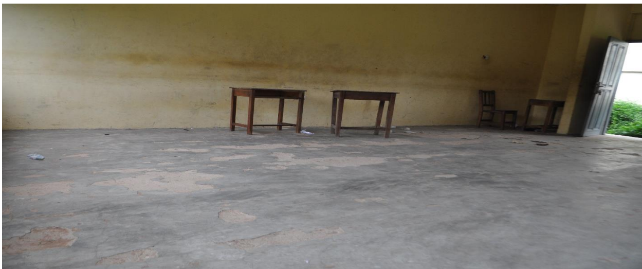
Figure 28: State of 6-Unit Classroom Block at Bishop Herman SHS
