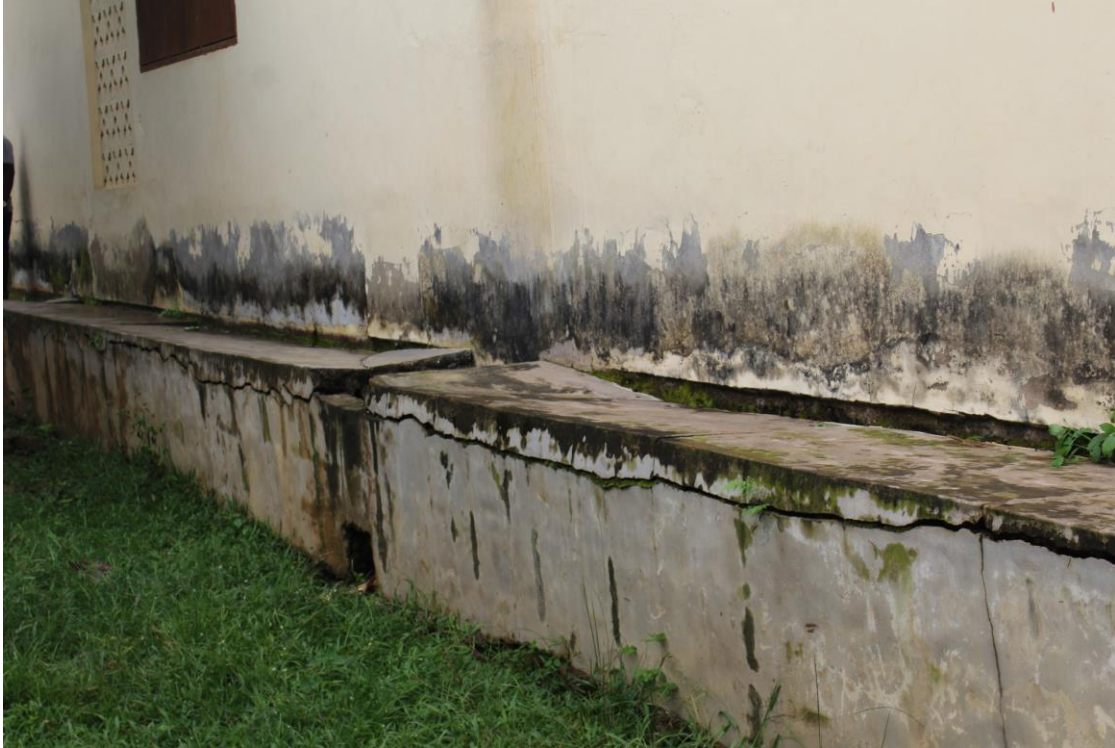
Figure 20: 6-Unit Classroom Block at Apedwa SDA Primary School Showing Serious Signs of Damage
