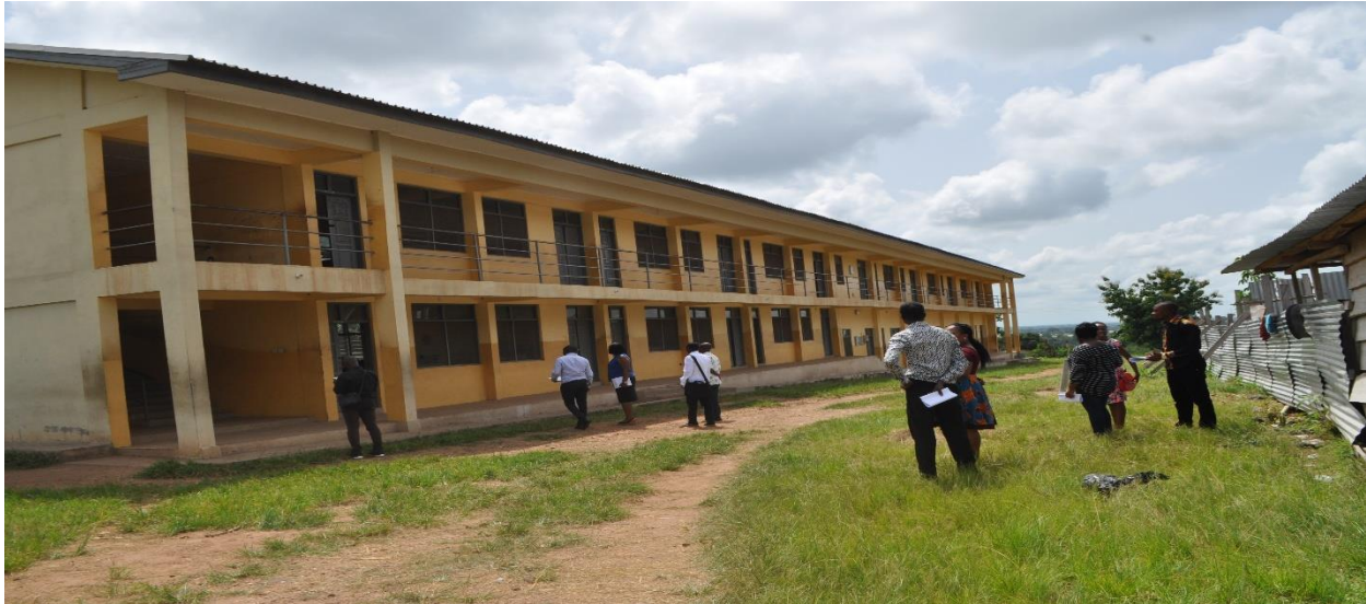
Figure 24: State of 2-Storey Dormitory Block at Mawuli SHS
