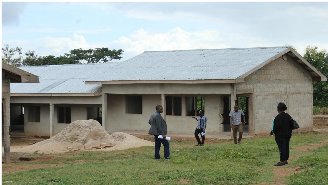
Figure 16: State of Agogo Saviour D/A Primary School
