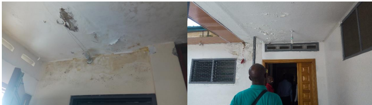
Figure 23: Renovated Headmistress' Bungalow Showing Signs of Deterioration from Leakages
