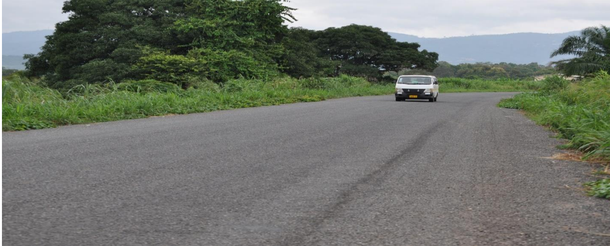
Figure 9: State of the Have-Kpando Road
