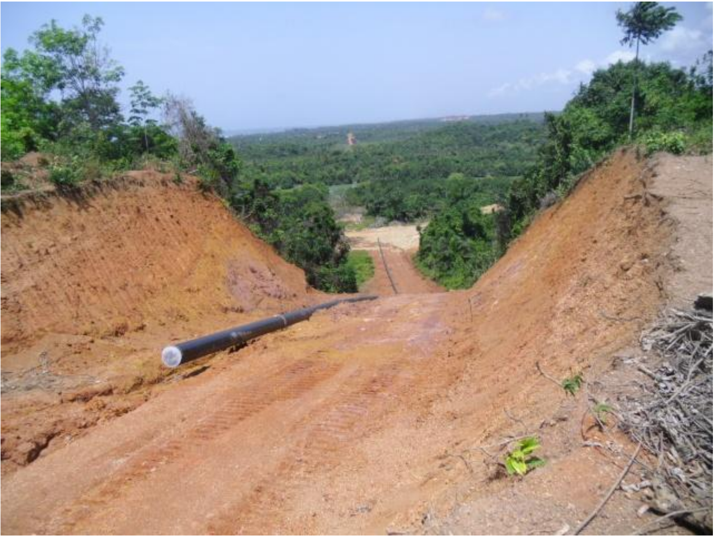
A gas pipeline being laid at the Ghana National Gas project site
