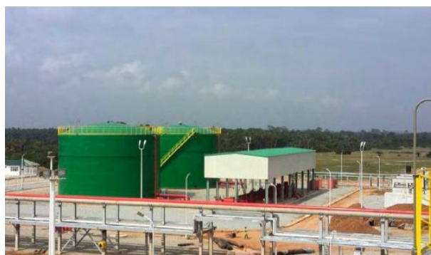
FIGURE 1: OVERVIEW OF WATER FIRE TANKS
