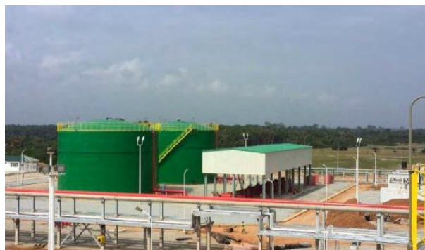
Figure 1: Overview of Water Fire Tanks
