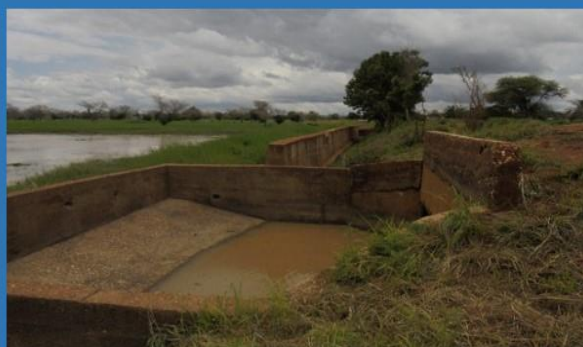
State of Duori Dam in the Upper West Region
