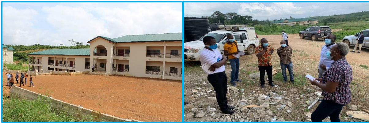
The PIAC team inspected ongoing works at the Anomabo Fisheries College in the Central Region.
