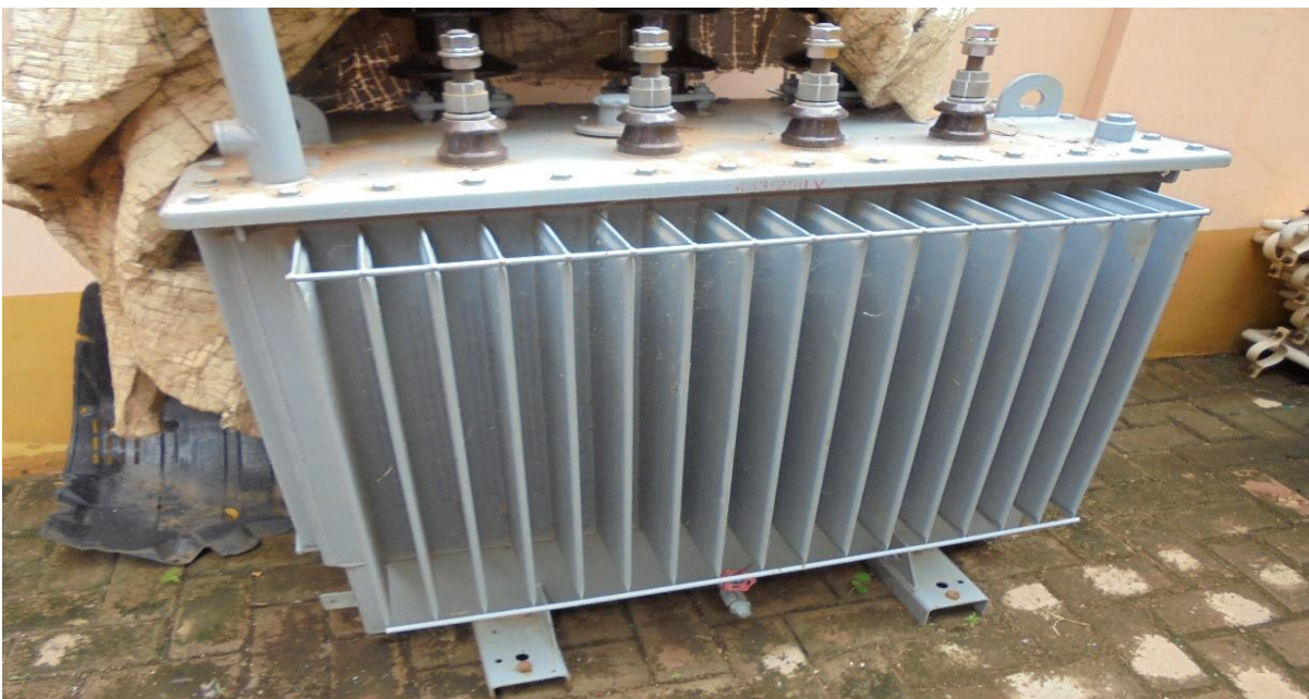
Figure 7: Transformer lying idle at administration block of Bagabaga College
