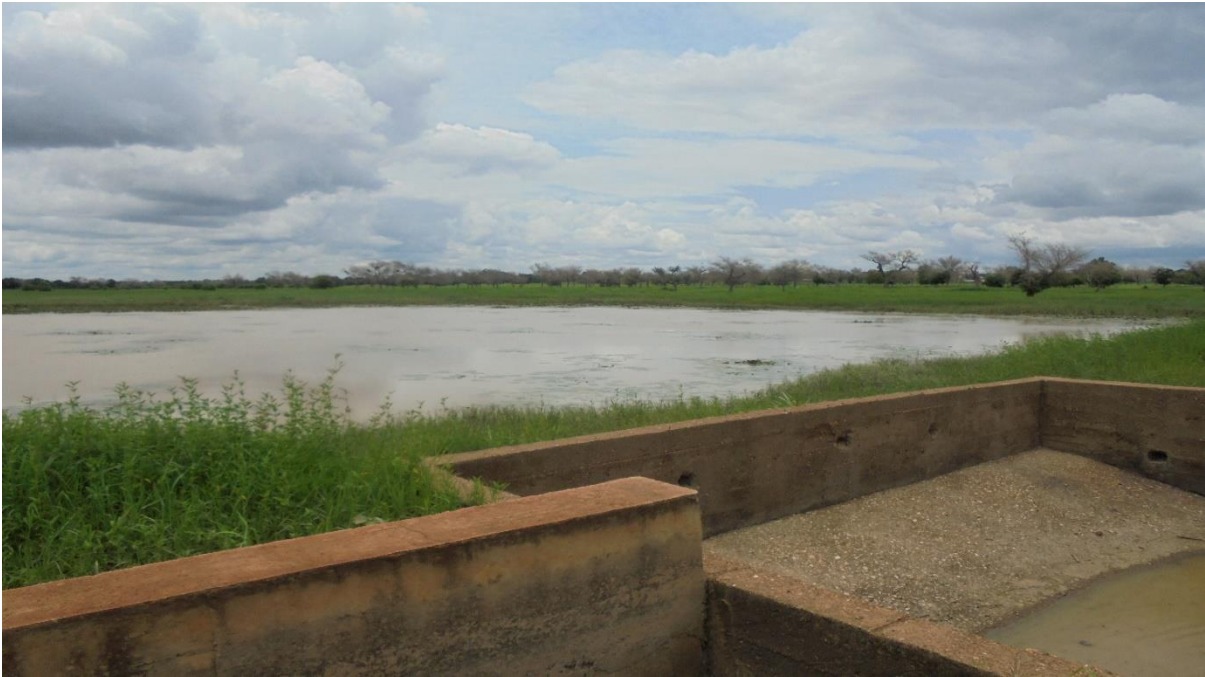
Figure 4: State of Douri Irrigation Dam in Upper West Region
